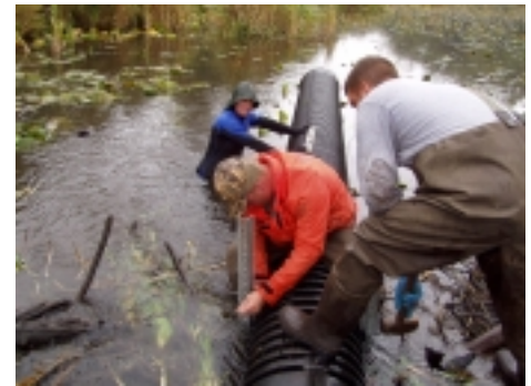
Leveling and adjusting rigid pipe in the breach of the dam to achieve the desired water level.
