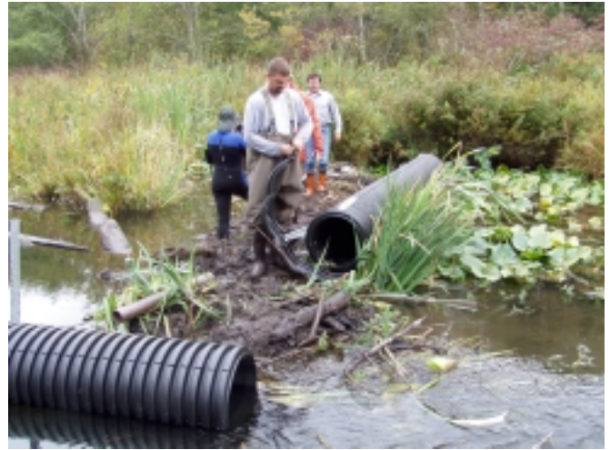
Installing and coupling rigid pipe in a breached beaver dam. Photos courtesy of Skagit County.
